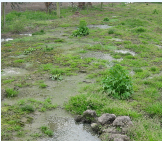
Failed soakage field
