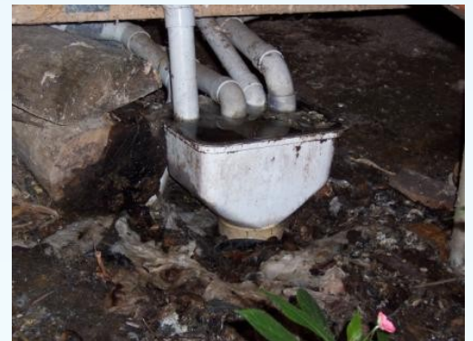
Backup to gully trap from clogged tank
